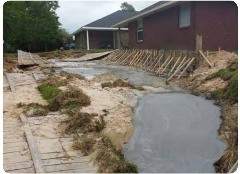
April 2014 flood damage - Newcastle
